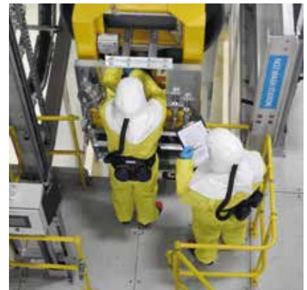
Tails Management Facility Capenhurst, UK
