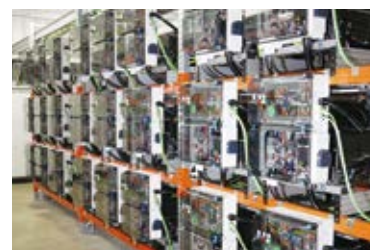
Large energy storage system operated by The Mobility House
