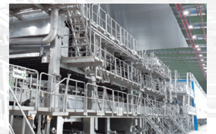
The production plant under construction at KRAFT OF ASIA PAPERBOARD & PACKAGING CO., LTD
