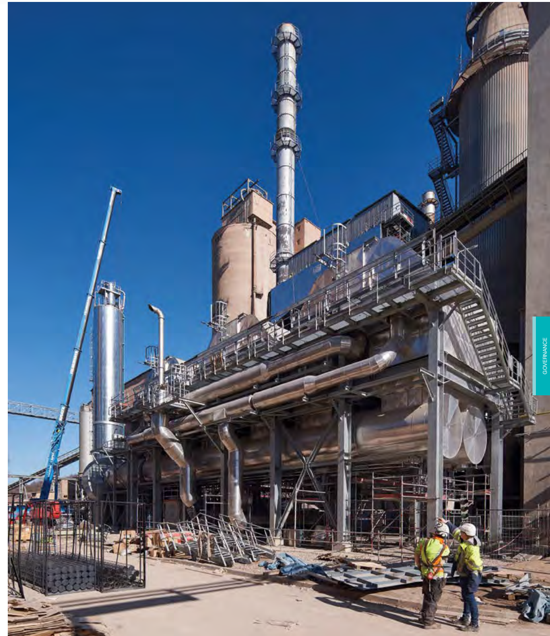
In July 2019, OPTERRA, part of CRH's Europe Materials Division and one of the leading cement producers in Germany, officially inaugurated a new exhaust gas purification system at its Karsdorf cement plant near Leipzig. The new filter technology, which includes a state-of-the-art AUTONOX ® Low Dust System installed on the existing kilns, enables the factory to comply with new limits for dust, ammonia and nitrogen oxide emissions.
