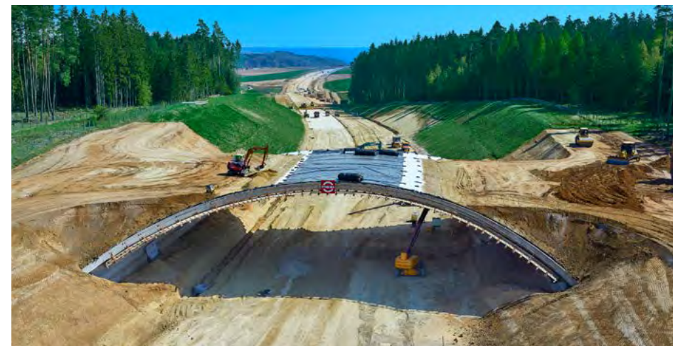
OPTERRA, part of CRH's Europe Materials Division, supplied concrete for this 'green bridge' on the Bundesstraße motorway project in Southern Bavaria, Germany. The project, which runs through a forest area, includes a new motorway as well as 14 additional structures. The green bridge, completed in May 2019, will enable wildlife to cross the busy motorway, thus reducing the impact of the project on the area's biodiversity.
